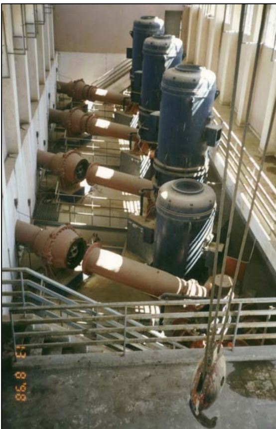
Main Pumping Station
